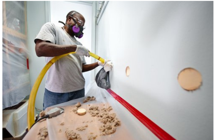
William Stewart, A Member of Veterans Green Jobs, Blows Cellulose Insulation into Interior Walls.
